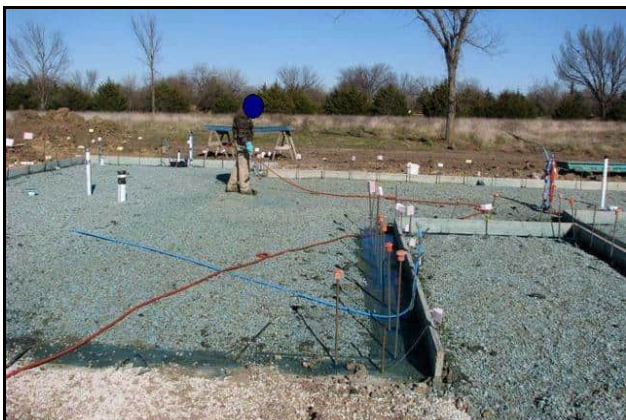
Above: After the interior final grade is established, the applicator applies termiticide to the flat surface over which cement will be poured.
