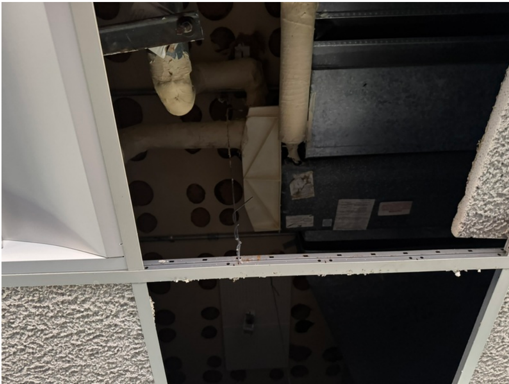
11. TSI and mastic from acoustical tiles
