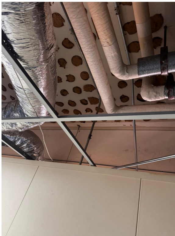
10. TSI and mastic from acoustical tiles
