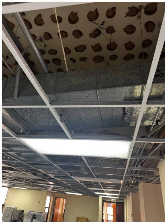
6. Mastic remaining from acoustical tiles
